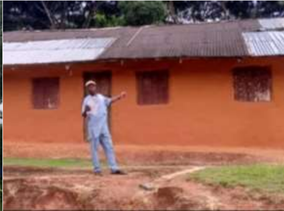
Plate 2: Corroded Mud House
