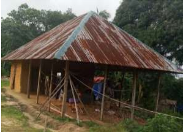
Plate 1: Rusty Open Shelter
